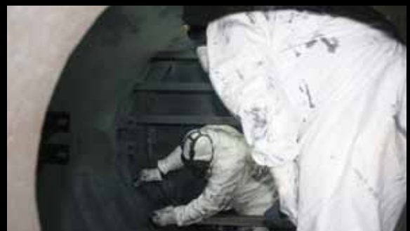
Rubber Lining Ion Exchange Vessel for NZ Refinery
